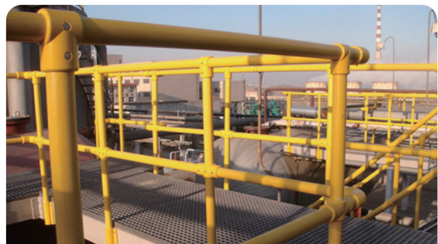
Round Handrails Platform
