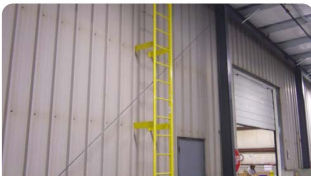
FRP fixed ladder for roof access.
