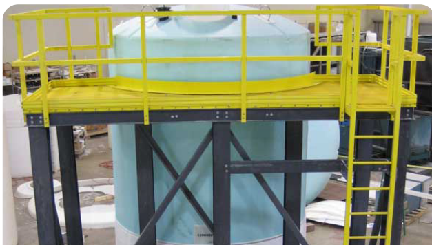
FRP fixed ladders for platform access
