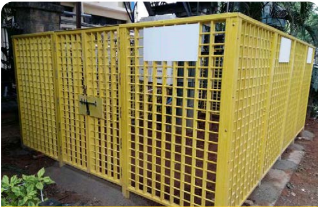
Electrical Substation Guardrail
